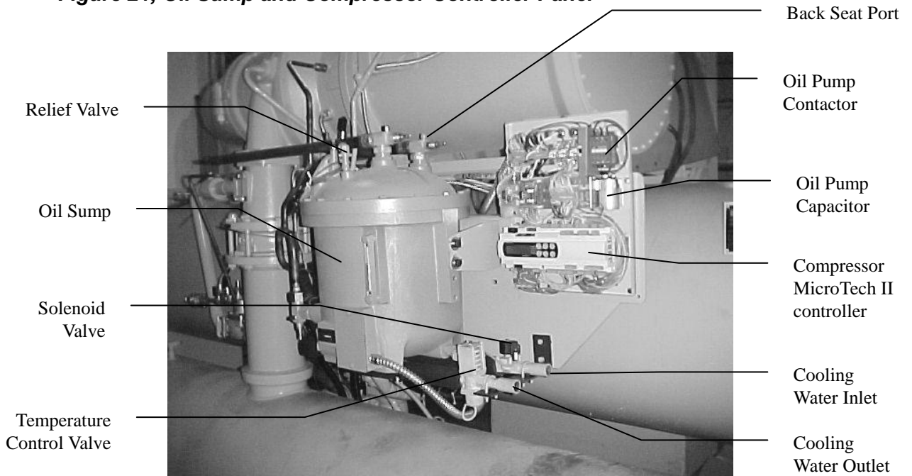
Figure 21, Oil Sump and Compressor Controller Panel
